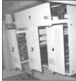
[C/B Rack Structure]
